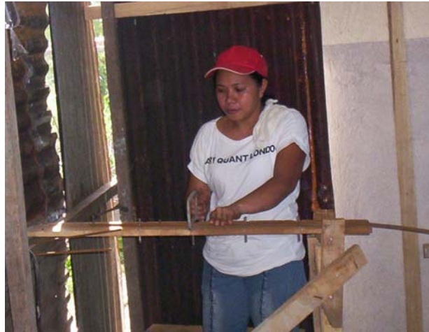
Gina Sanchez, 33, cuts a steel bar to be used as a beam in one of the houses of a new community. Her labor earns equity in a home she will own with her husband and four children in Butuan City, Philippines.
